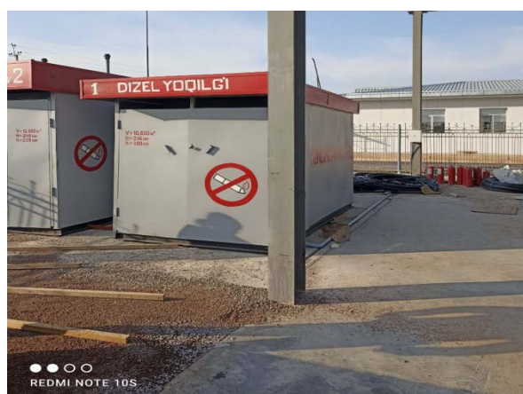
Tank for storage of oil products
