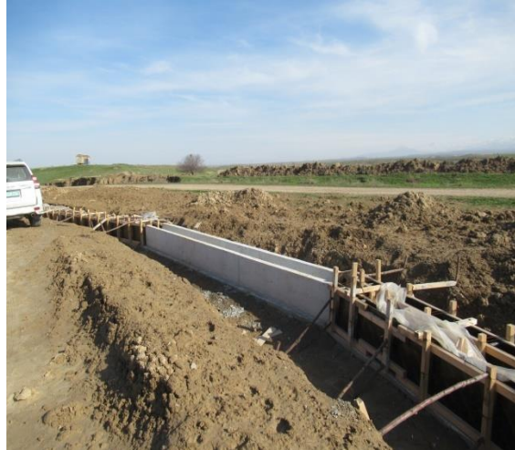
Pic. 8 Pouring a concrete pallet in the administrative part of the facility (09.06.2023)
