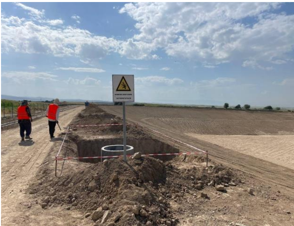
Pic. 1 Safety fence and warning sign (10.09.2023)
